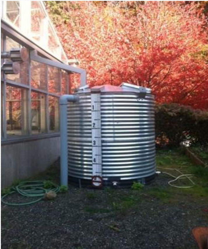
1,000 gallon tank near Biology greenhouse
