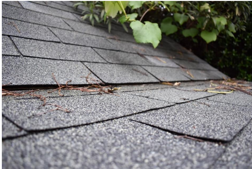
Figure 1: Traditional asphalt fiberglass shingle roofing makes suitable potable rainwater catchment surfaces. However, users should avoid algae-resistance treatment and purifying their water with chlorine. [By FASTILY [CC BY-SA 4.0 ( https://creativecommons.org/licenses/by-sa/4.0/ )], from Wikimedia Commons]
