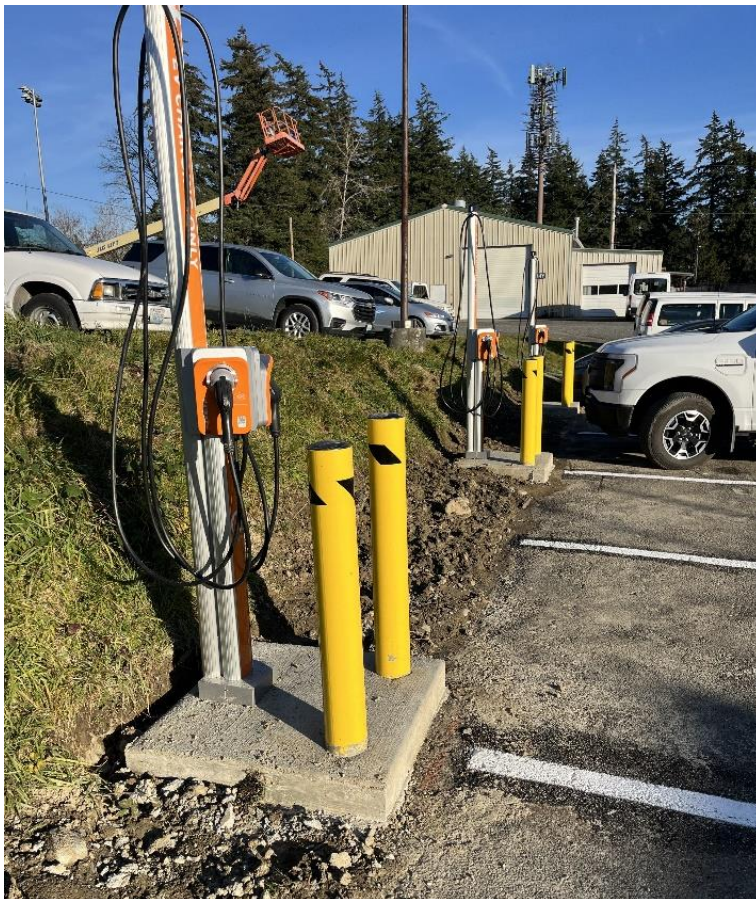
Pictured: new electric charging stations in the Physical Plant parking lot. Source: FDO
