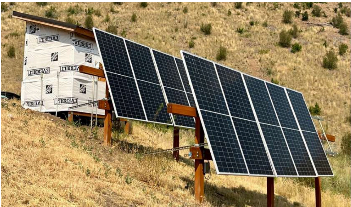
Figure D: Secondary view of Stacey Mathew’s solar power system.
