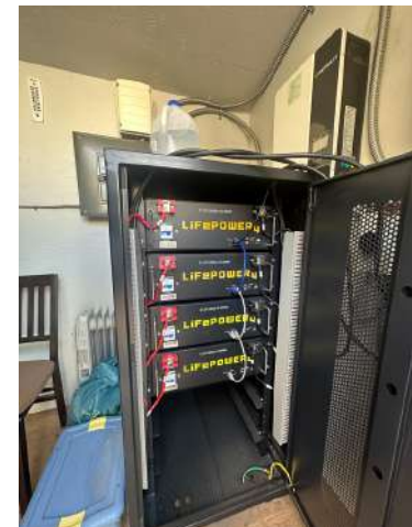
Stacey Mathews' solar battery set up.
