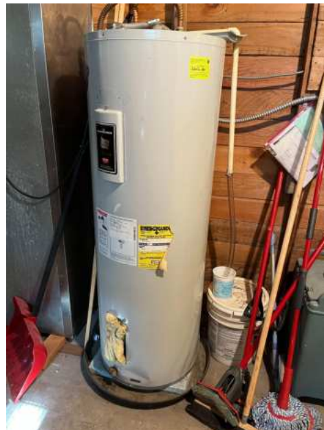
Current water heater at Twisp Valley Grange Photo by Olivia Palmer
