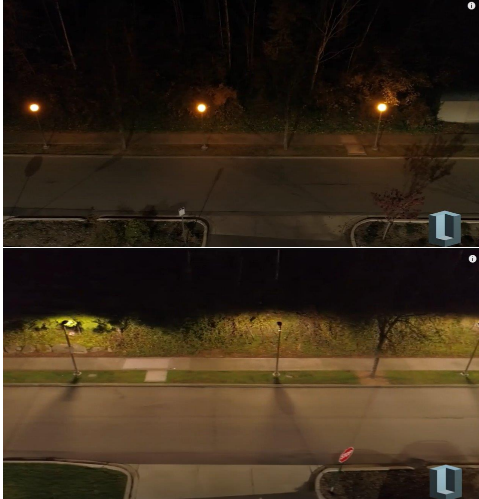
Before and after photos of LED lighting retrofits described in objective 1.3 and 2.3. (Photo source: FDO)
